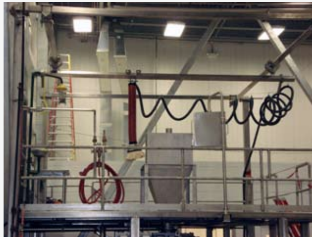
Stainless steel sack lifter unit installed in a juice manufacturing process.
